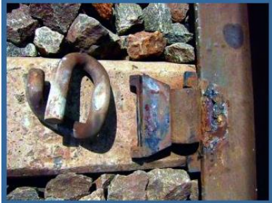
Field sample showing corrosion under liner http://home.iitk.ac.in/~vyas/tmrs/P2a.html
