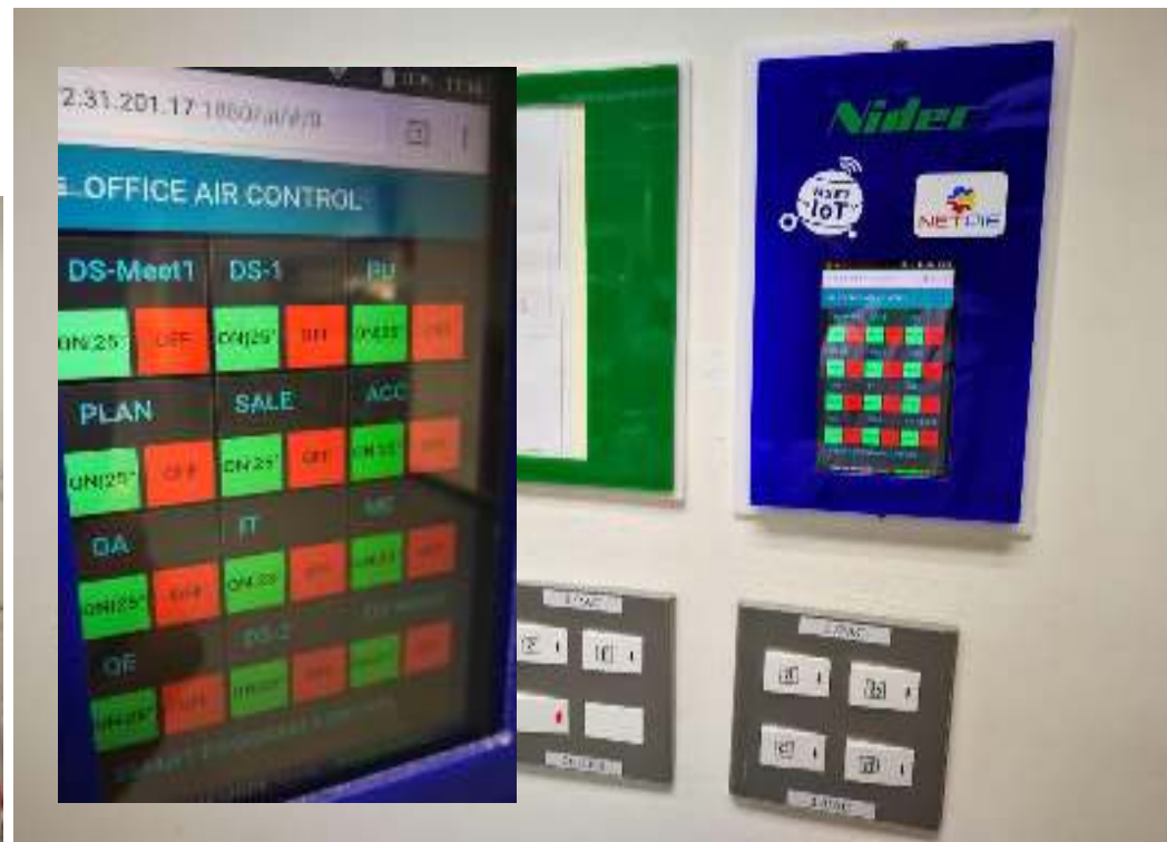
Air Conditioners Center Control (Office Area)
