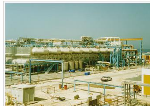
MSF Desalination Plant at Jebel Ali G Station, Dubai
