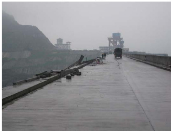
Figure 11 Dam crest of Zipingpu CFRD after the quake
