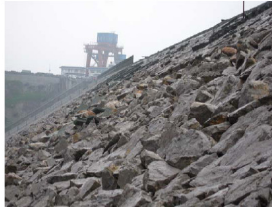
Figure 14 Settlement and loose rockfill on downstream slope
