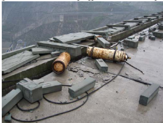
Figure 12 Collapsed banisters and the crack of downstream crest
