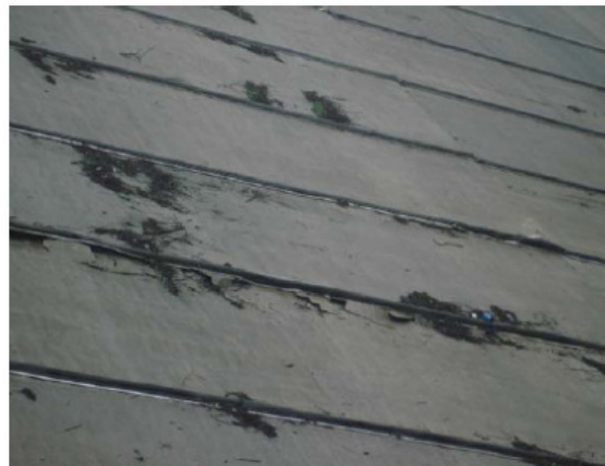
Figure 15 Rupture of upstream face slab
