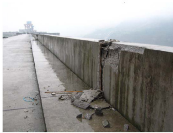
Figure 13 Rupture of the parapet wall
